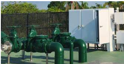
Water Pump Stations
