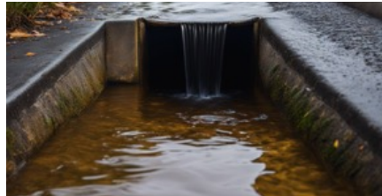
Stormwater Control Structures
