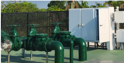
Water Pump Stations
