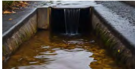
Stormwater Control Structures
