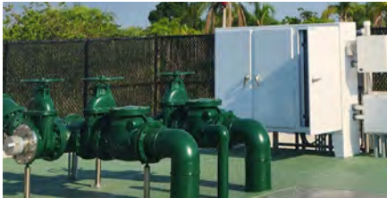
Water Pump Stations
